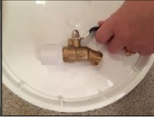
Figure 6 The hose bibb screwed into the PVC bushing.
